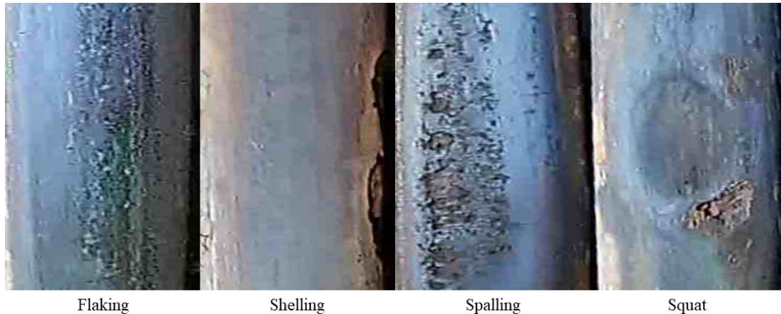
Figure 1: Prominent Rail Surface Deformities
